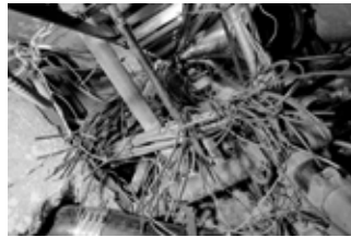
An original electrical shaft in the Multnomah County Courthouse
