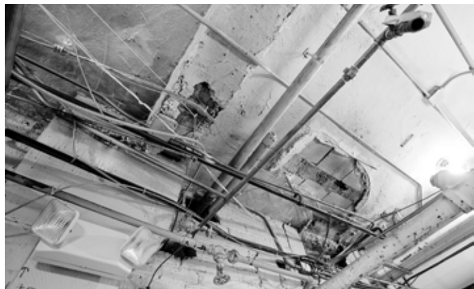
Patchwork of electrical, plumbing and exposed masonry
